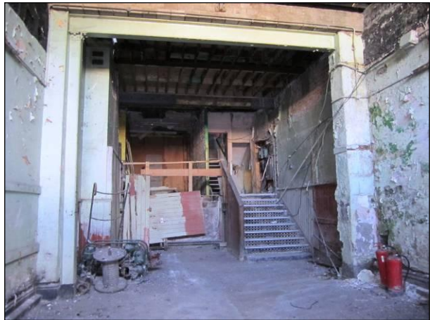
View E of ground floor of former fire station. The cross beam marks the beginning of the original house.
