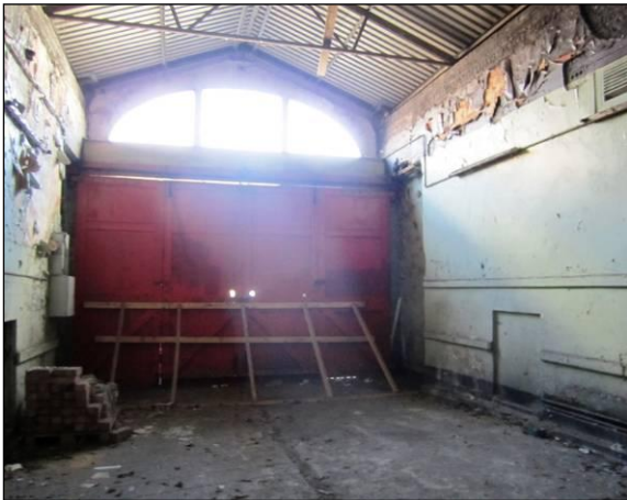
View W of ground floor of former fire station to front of main house.
