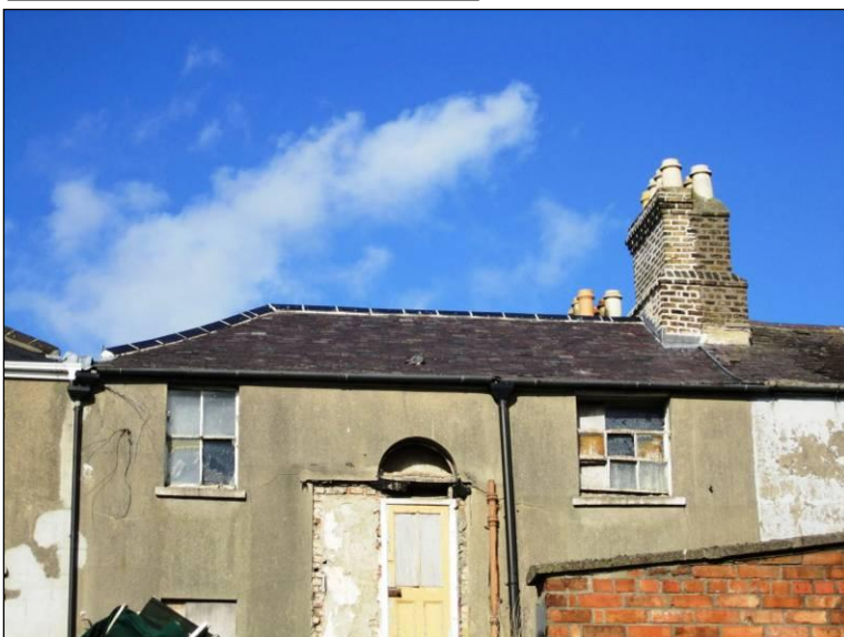
View of rear elevation of main house and detailed view of Blue Bangor slate roof.
